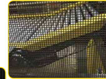
Emergency Product Exit From Tunnel When Downstream Conveyor is Full
